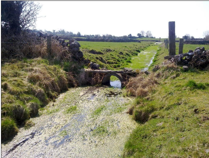
Photograph 24 – Typical Culvert along the Aggard Stream which requires replacement
