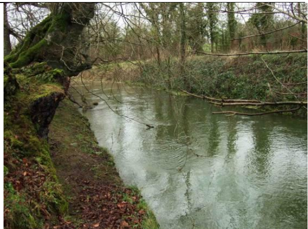
Plate 62: View d/s from AG6 - left foreground is toe of stepped drainage embankment (8-1-2012)
